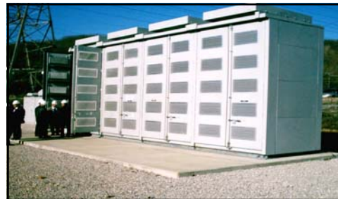
NGK 1.2MW / 7.4MWh NaS Battery Installation at AEP, Charleston, WV. Photo © John Baker
